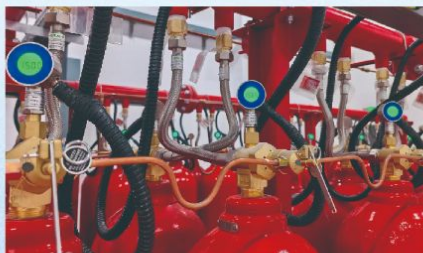
Smart Fire Protection
